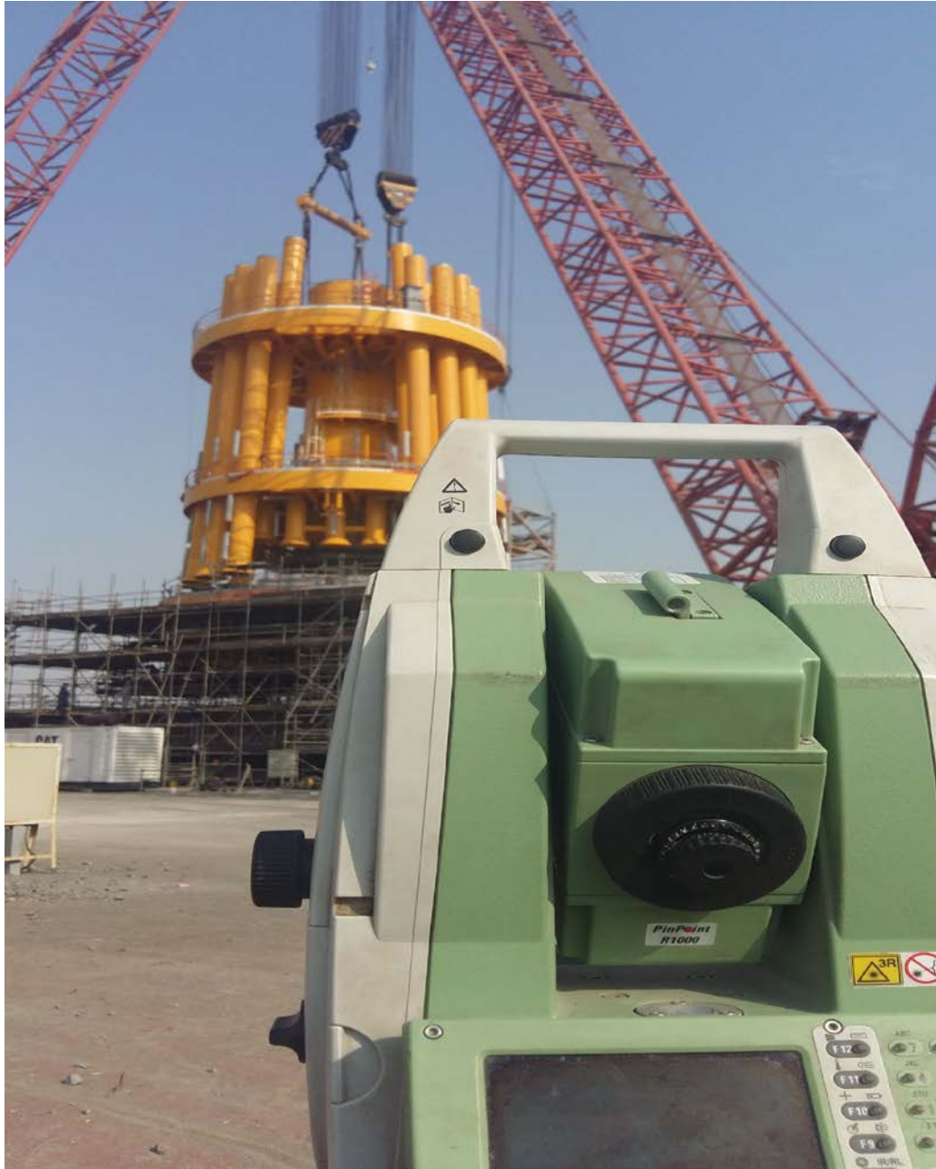
Leica TDRA6000 INDUSTRIAL TOTAL STATION used to measure Chain Table Fit-up after welding.
